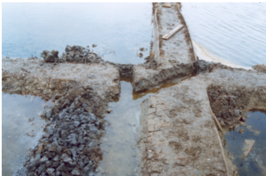
Figure 34 - Temporary circulation system
